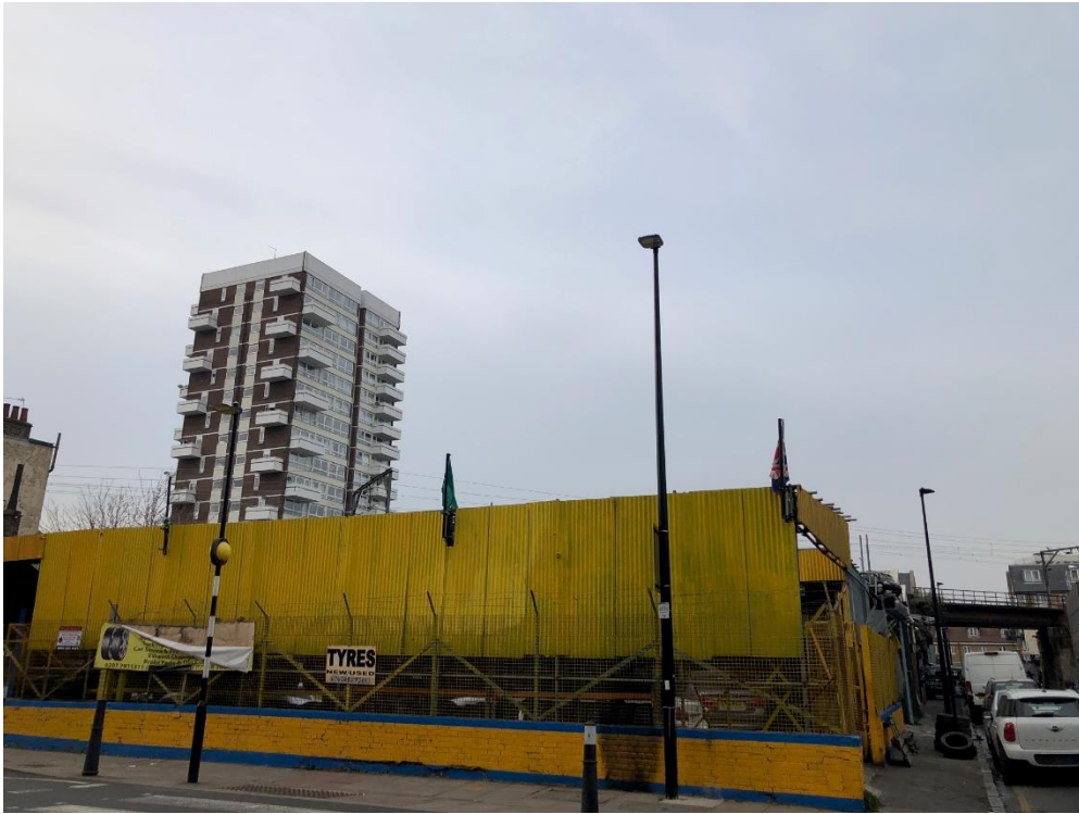
View from Salmon Lane looking North with Blount Street on the right of this image. Darnley House is the visible tall building which is 17 storeys of residential flats.
